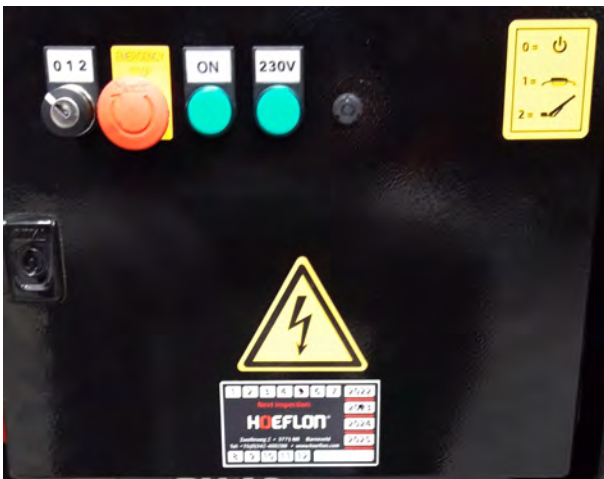
Figuur 2.5 Electrical cabinet exterior
